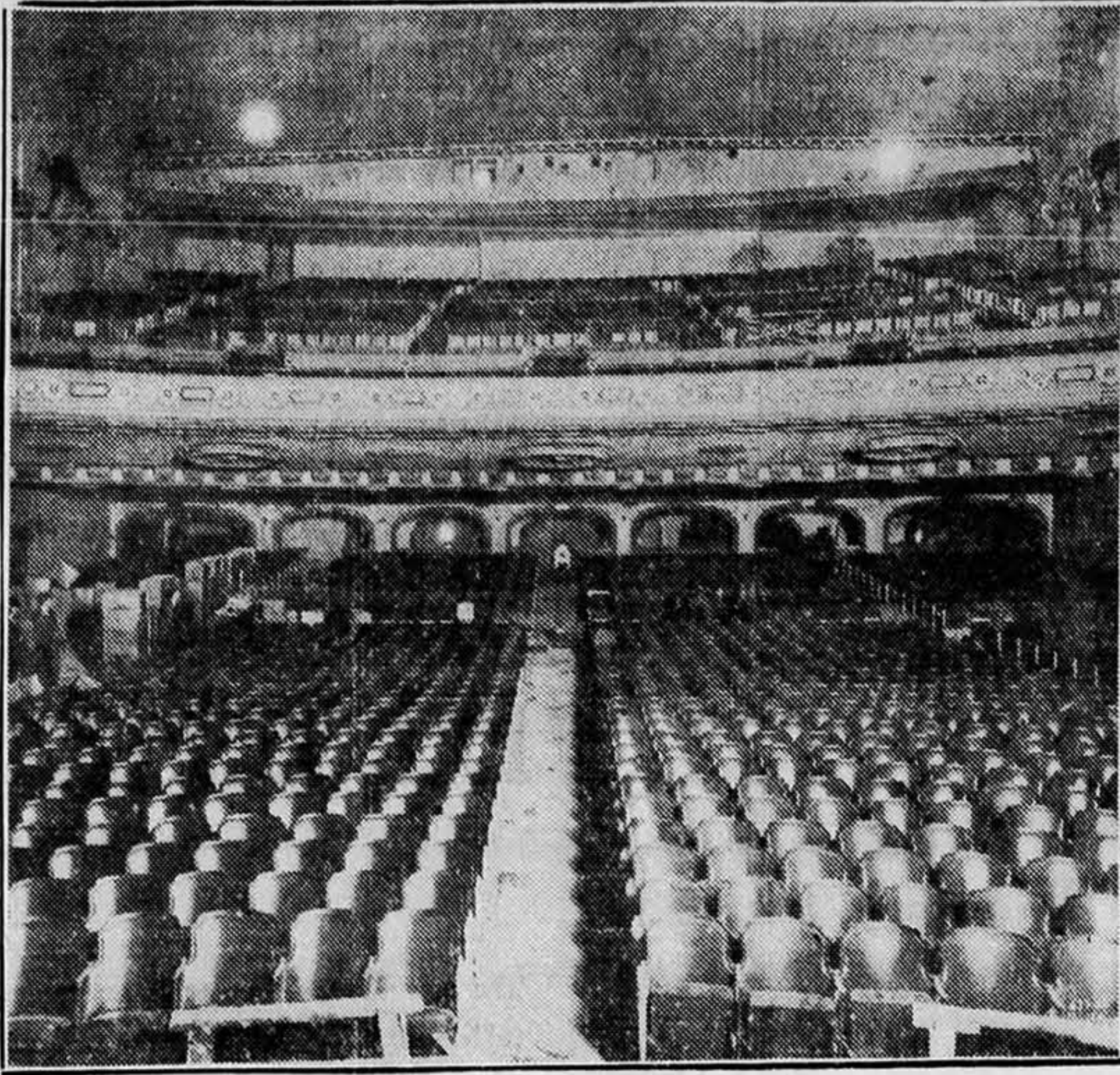
This photo taken during the last minute rush to install seats in the new Loew's Akron gives the reader an idea of the size of this beautiful playhouse. Loew's Akron seats 3,500.
