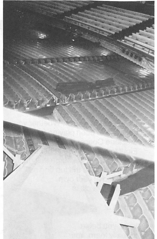
NOT FOR KIDS—In the course of organ installation a builder is called on to perform a myriad of jobs not normally associated with the actual job of erecting an instrument. In Pasadena Civic Auditorium, Builder Junchen had to build two ramps to pull heavy components into the chambers. One is shown here.
