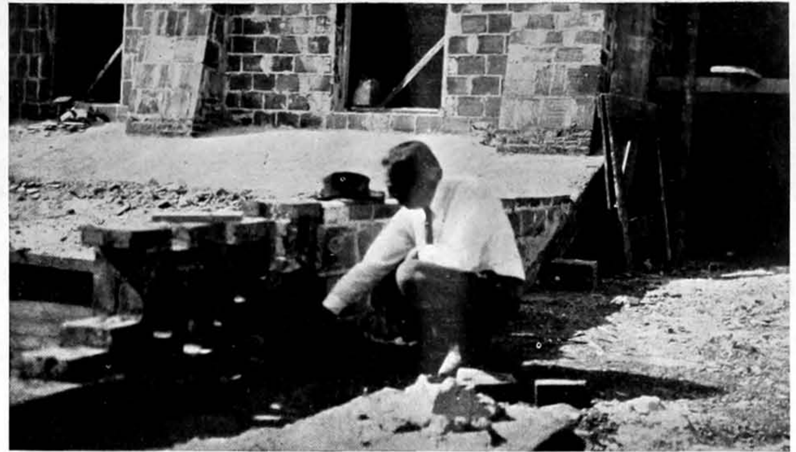
CONCRETE AND BRICK CAN BE MADE BEAUTIFUL. MR. ALSON CLARK SETTING THE BRICKS FOR THE GRILL AS HE HAD SEEN ONE IN MEXICO.
