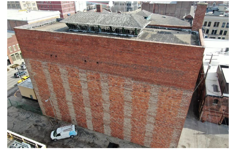
EXPOSED CLAY TILE WEST FACADE
