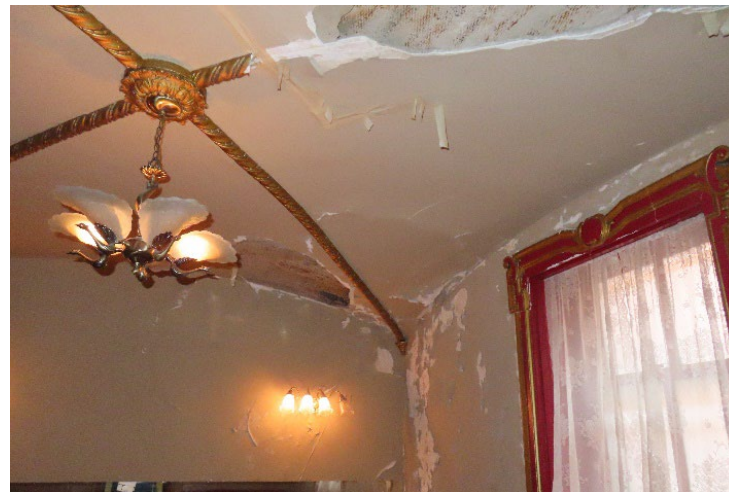
MISSING PLASTER, EXPOSED LATH, + PEELING PAINT
