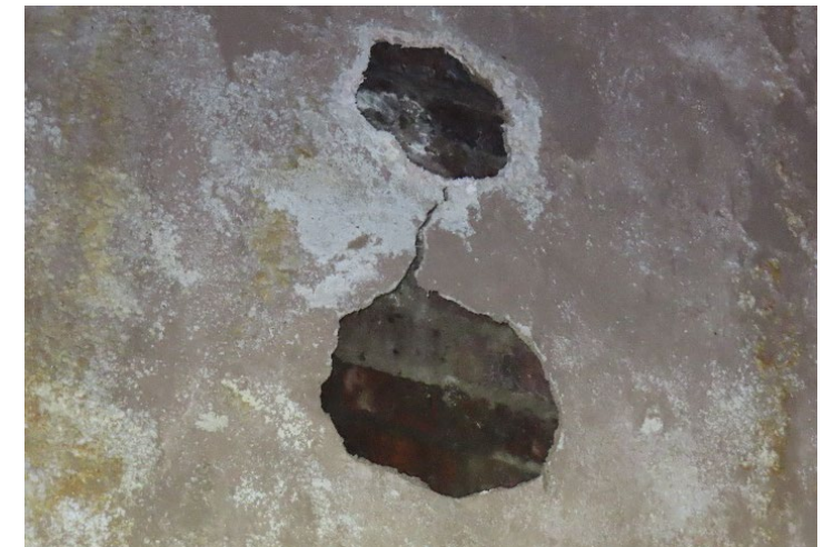
MISSING COATING, MISSING PLASTER, + EXPOSED BRICK BACKUP
