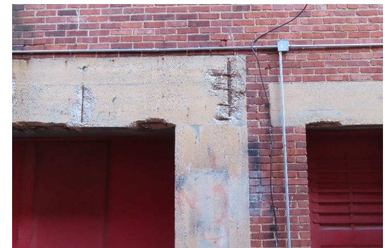
SPALLED CONCRETE LINTELS + DOOR FRAMES
