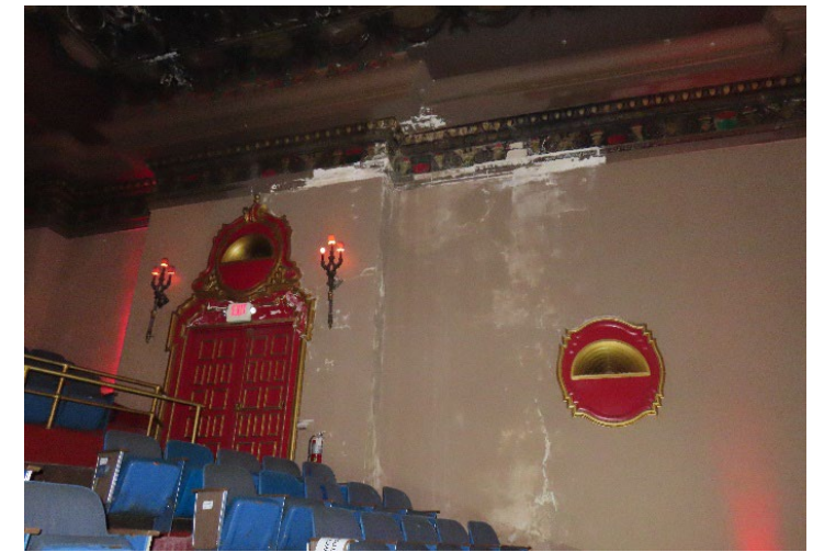
WATER DAMAGE ON WALL + CEILING
