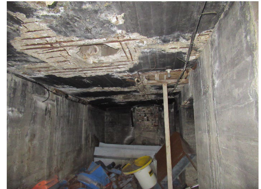
SPALLED CONCRETE + EXPOSED REINFORCEMENT IN BASEMENT AREAS
