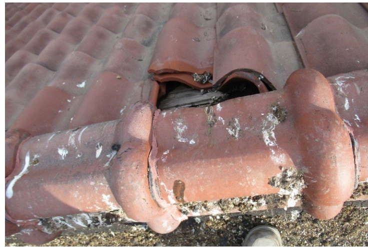
CRACKED + MISSING TILES
