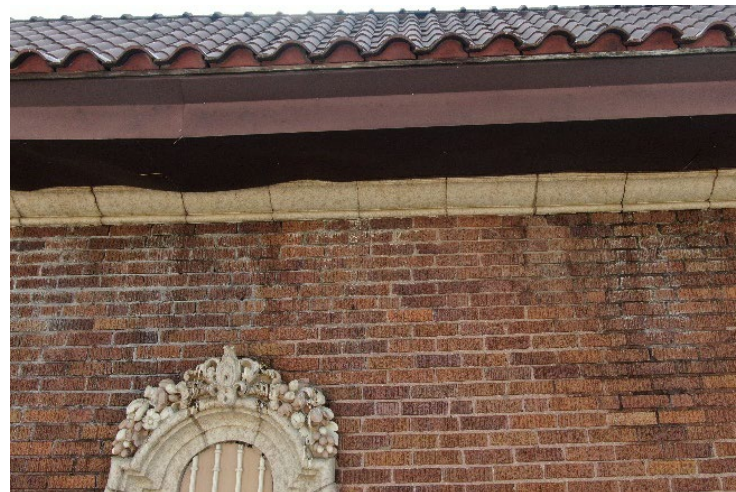
MISSING GUTTERS + STAINED FACADE
