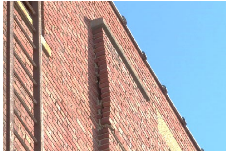
DISTRESSED PILASTERS SOUTH FACADE
