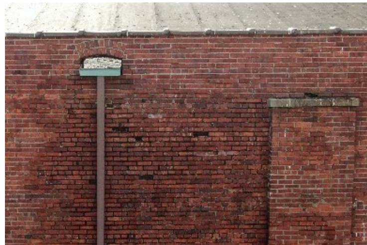
DETERIORATED / STAINED BRICK
