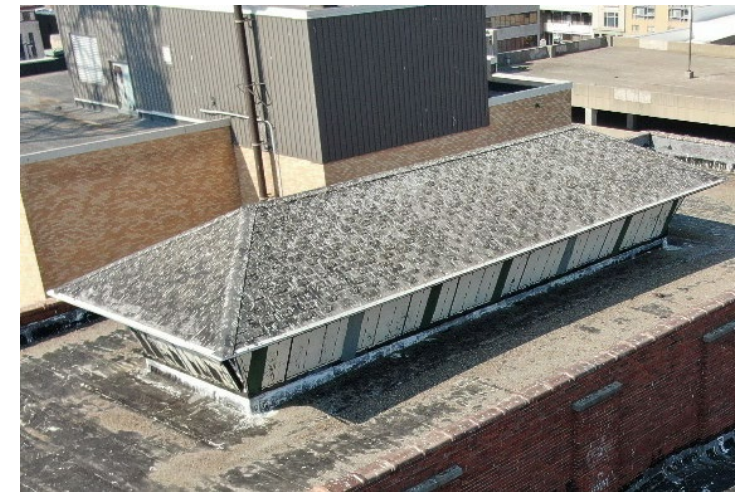
FRIABLE + MISSING SHINGLES
