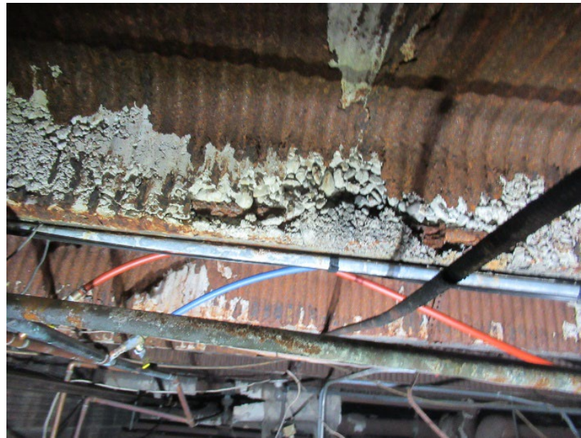
CORROSION ON METAL CONCRETE FORMS
