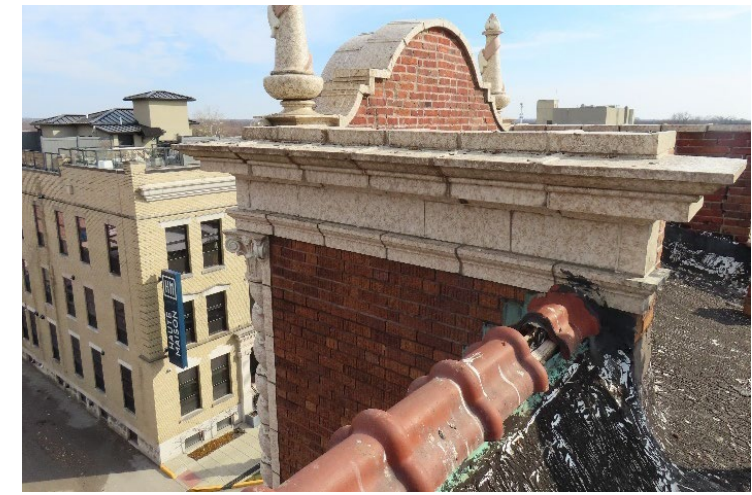
CRACKED, MISSING, OPEN COPINGS
