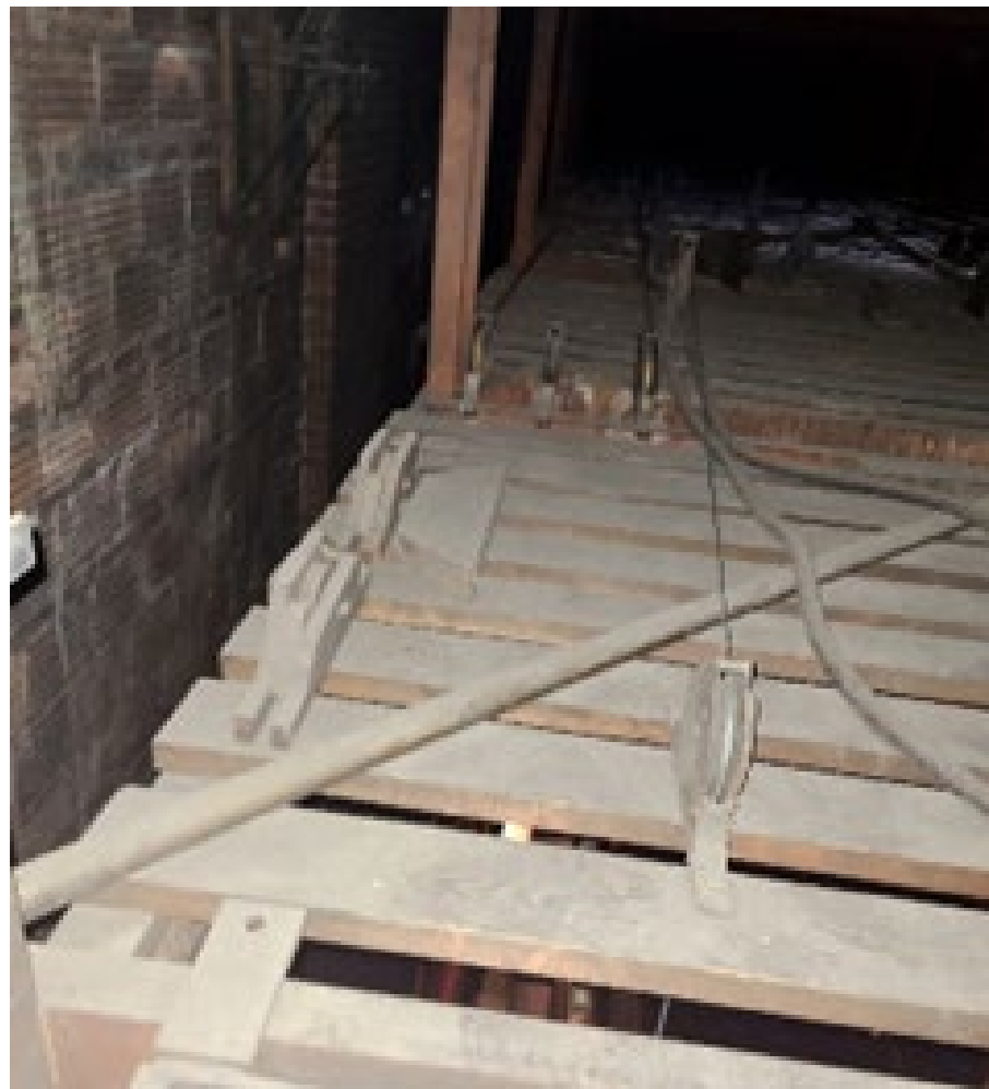
EXISTING GRID ABOVE STAGE
