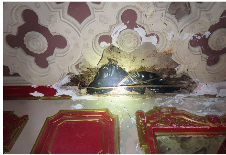
MISSING PLASTER EXPOSED METAL LATH
