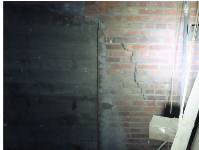
CRACKED BRICK TO PROSCENIUM ARCH
