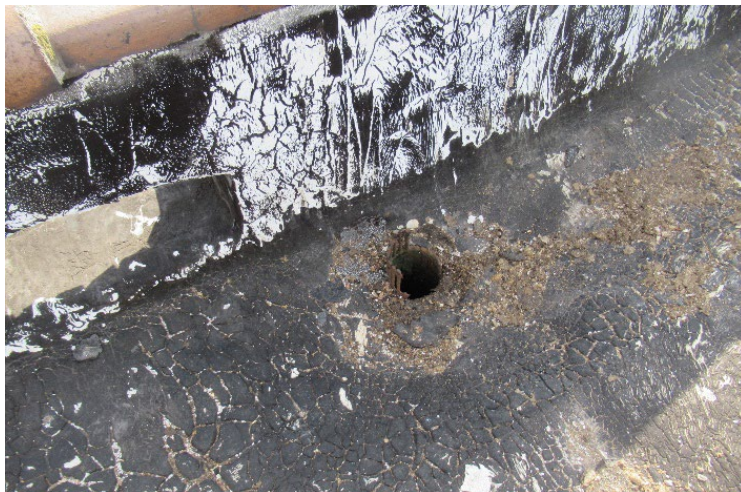
BROKEN / MISSING STAINER DRAINS
