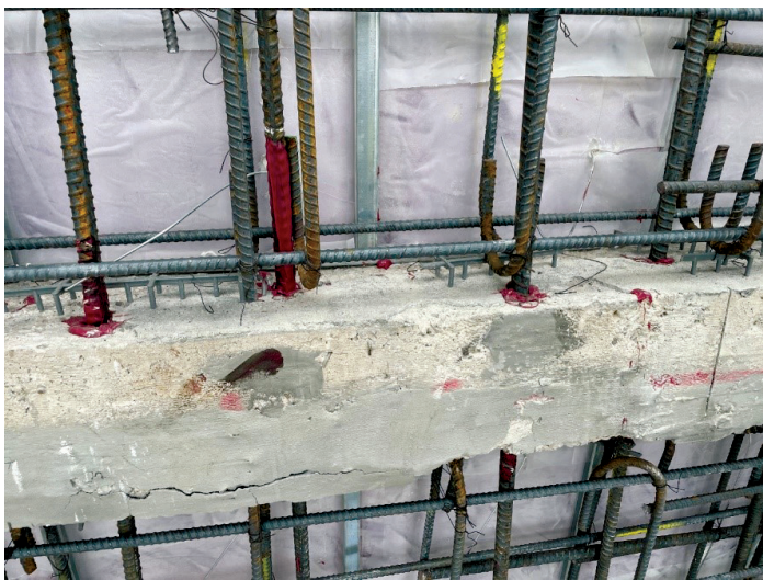
Fig. 4. During shear wall reinforcing, the installation of rebar dowels required frequent coordination despite the design considerations because the existing reinforcing proved challenging to avoid. Filling abandoned drilled holes as the drilling proceeded was important to avoid losing excessive capacity of the existing concrete members.
