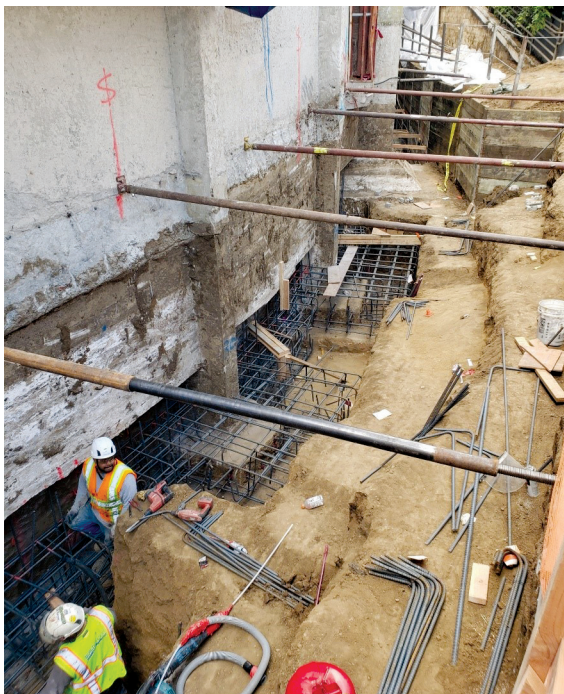
Fig. 6. Foundation construction required further coordination with the existing field conditions on a case-by-case basis; some steps that were previously assumed to be required were eliminated, and step heights were adjusted to reduce the number of steps as much as possible.
