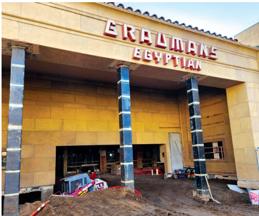
Fig. 7. After the portico columns were strengthened, they were analyzed to verify the plastic rotational capacity was adequate for the end rotations due to the inelastic building drift.
