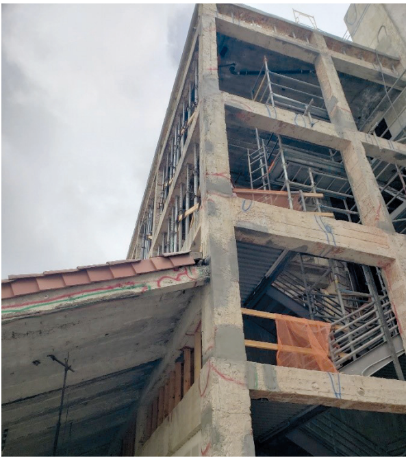
Fig. 8. Concrete frame repair at southwest portion consisted of shoring where required to remove and repair poorly placed concrete, mortar or epoxy injecting cracks, cleaning, and repairing corroded reinforcing, and placing repair mortar at spalls and to achieve proper clear cover on reinforcing bars.
