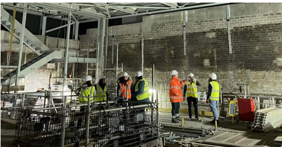
Works being done to increase the height of the fly tower roof
